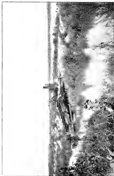
3. Supplementary engine and elevator for carrying water from dredge cut to pond, Monroe, Mich.
