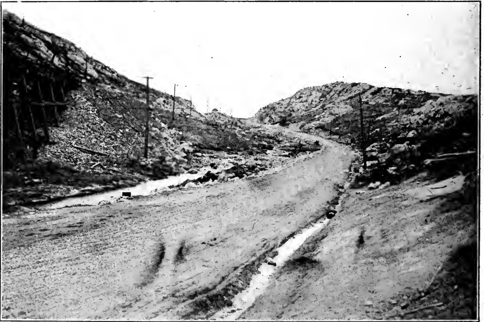
Sudbury and Murray Mine Stone Road passing under the Algoma Eastern Railway.
