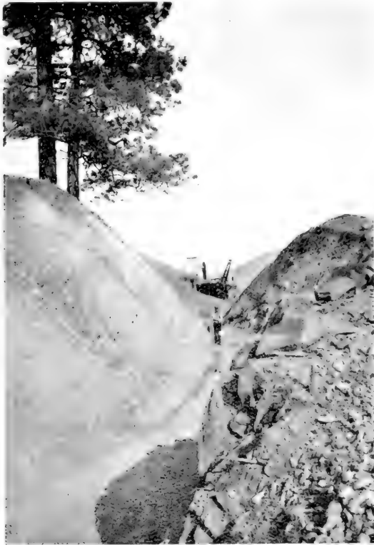
IRRIGATION SCHEME, BIG CUT ON COLDSTREAM ESTATE, B.C.
