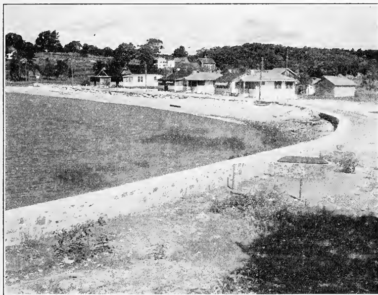
FIGURE 95. View at Shell Beach, Guilford, showing new sea wall and man-hole containing tide gate, built by relief labor.
