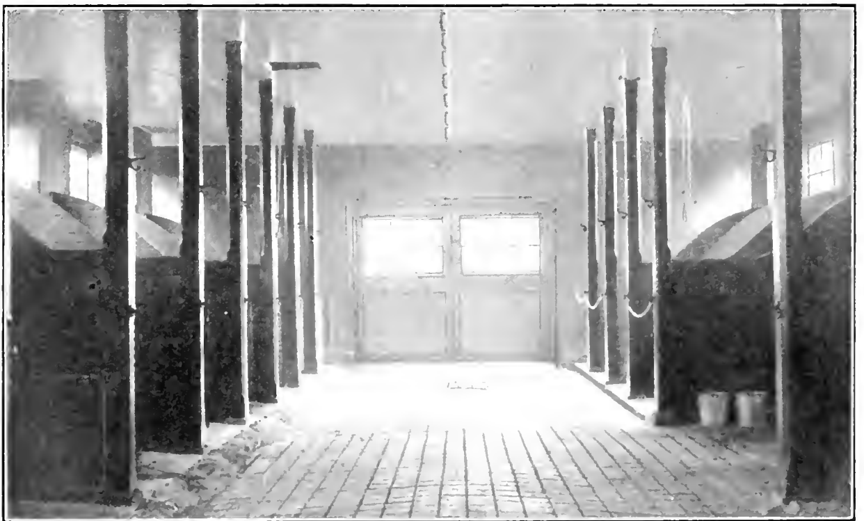
Interior View of Horse Stable, Cap Rouge, P.Q. Note the fresh air intake covered by grating in floor, and the foul air outlet in ceiling.
