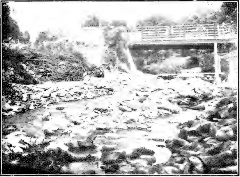
V. Mellte Castell bridge from South, showing debris left in the stream way by the flood. Note the dislodged supports to the bridge on the right.
