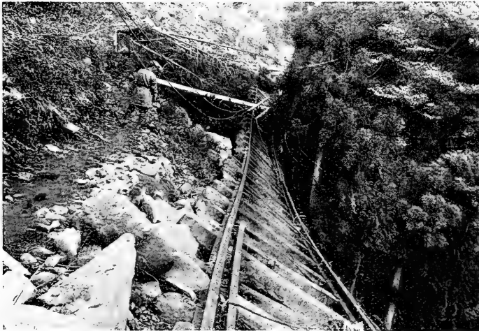
B. Damages due to land slides in the Hakone railway.
