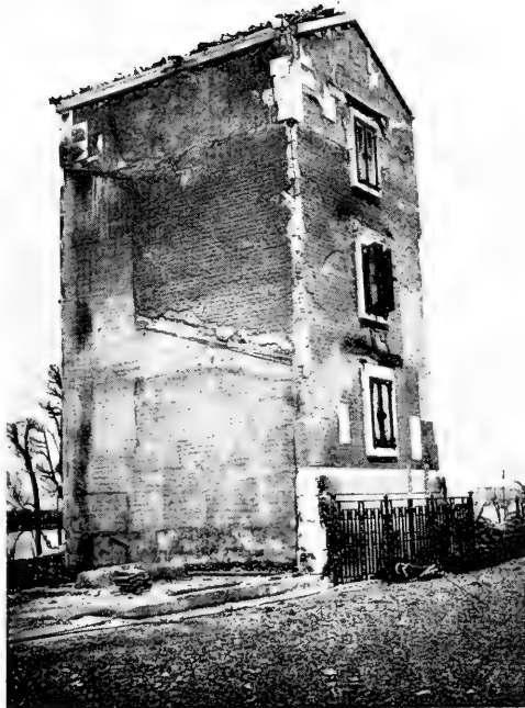
B. House constructed with porous glassy liparate withstood blazing fire. Things inside intact. (Hukagawa Ward, Tokyo.)
