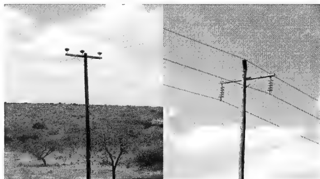
Figure 1a & b. 1a (on the left) shows the typical “T-structure” which poses an electrocution risk to birds perching on the cross arm. 1b shows the “inverted T” pole structure which is safer for perching birds since the outer conductors are suspended below the cross arm out of reach of birds.
