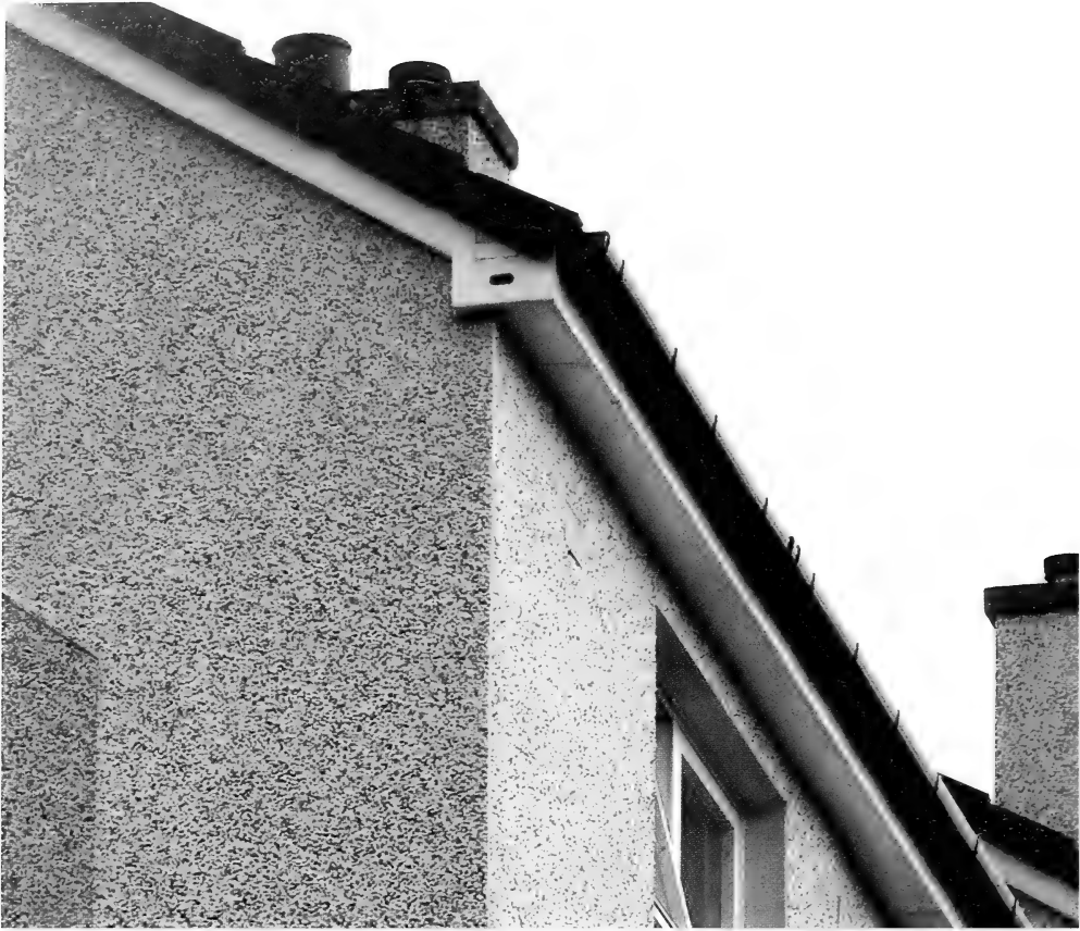
Plate 306. A hole cut in to the PVC soffit on the gable now provides a better design. © Clare Darlaston
