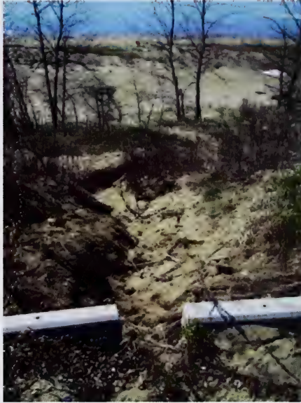
Figure 6. An example of erosion downslope from the pull-offs on the ridgeline.
