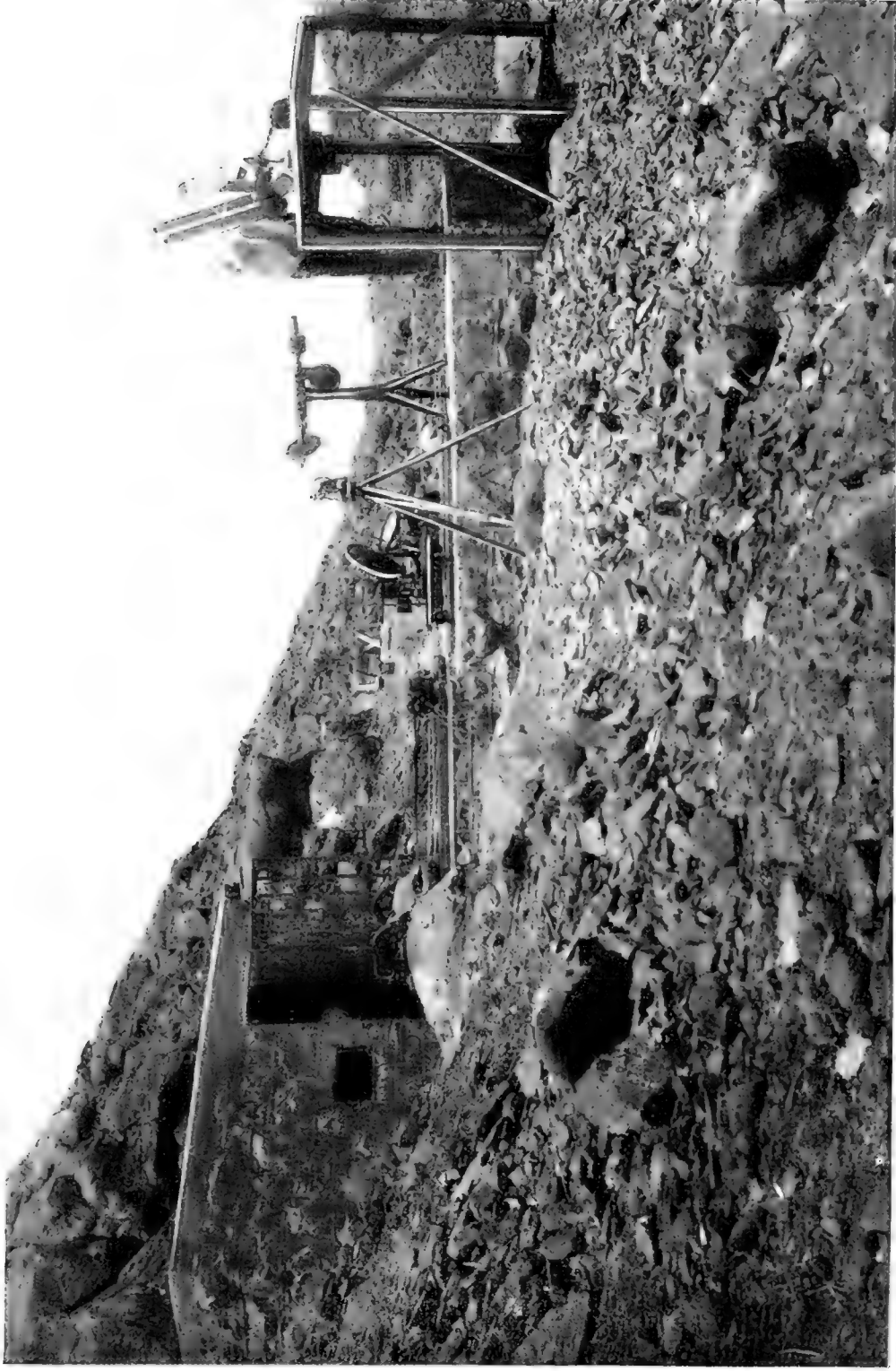
Observing tunnel and instruments for studying the variation of the sun's heat, on Mount Brukkaros, South West Africa. Established by the National Geographic Society
