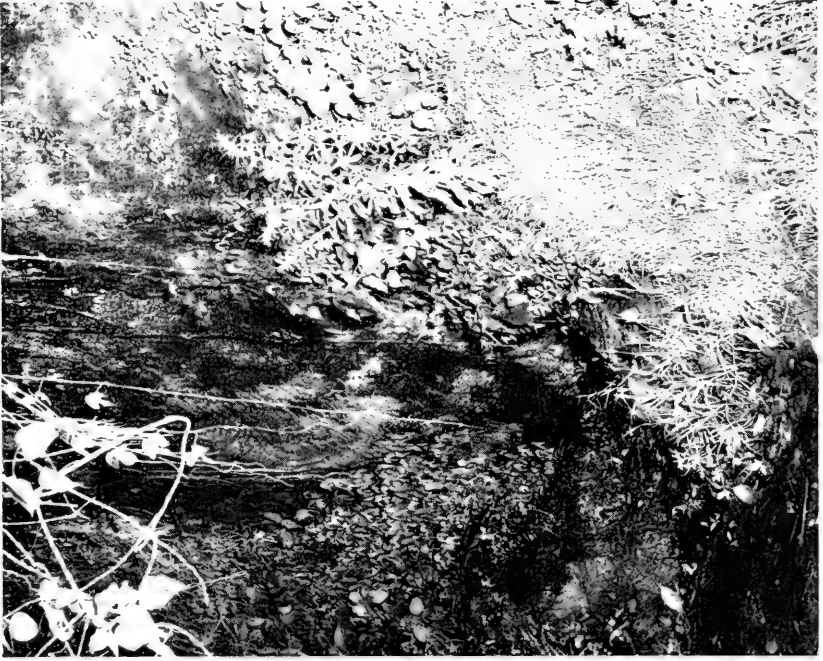
2. Flow from cavern cut out by constant drip along wet-faced wall.
