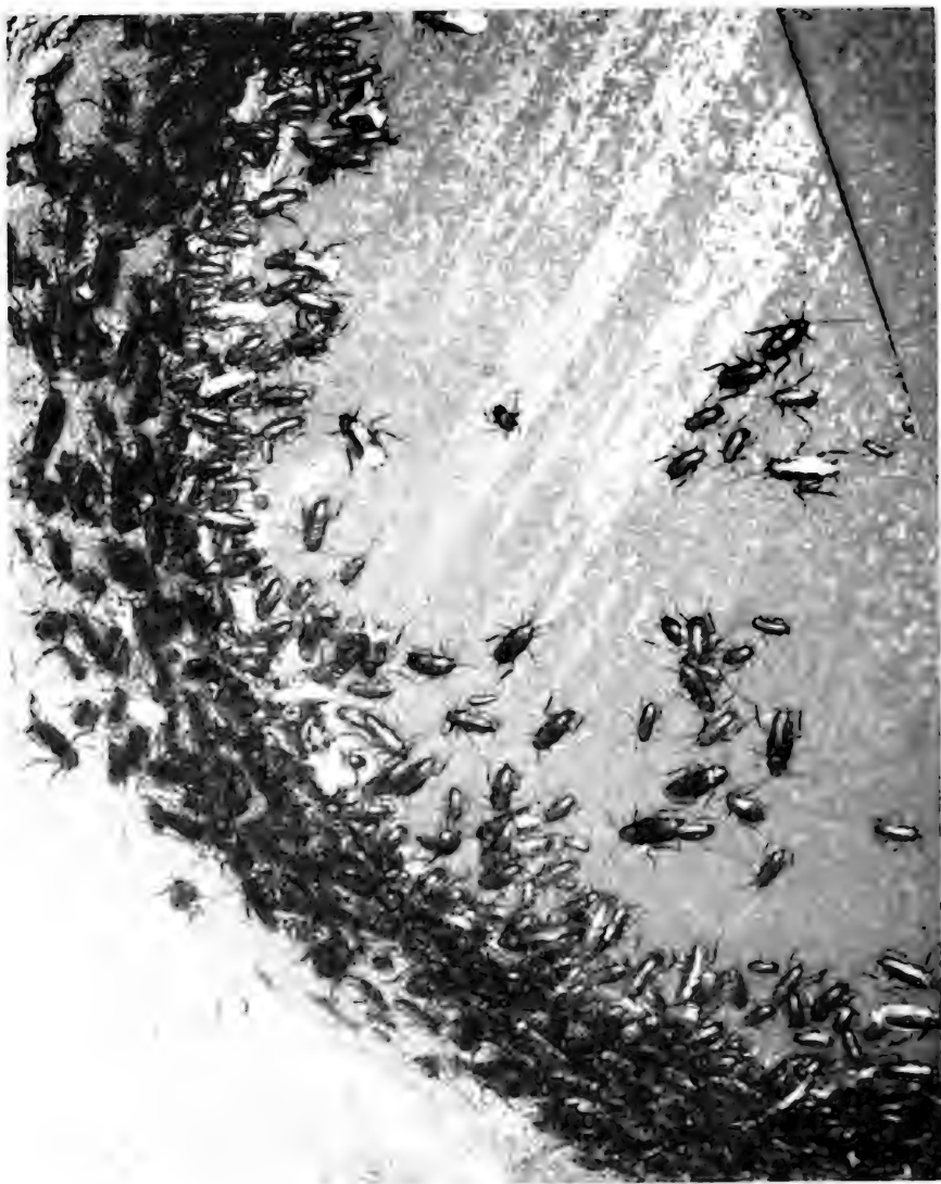
Periplaneta americana congregated on the arched roof and walls of a large sewer in Minneapolis, Minn. Approximately 3,000 cockroaches were present in a space of 12 square feet at the time the picture was taken. (See p. 11 for other details. Photograph by Jess Diggs and Alton Hollenbeck.)
