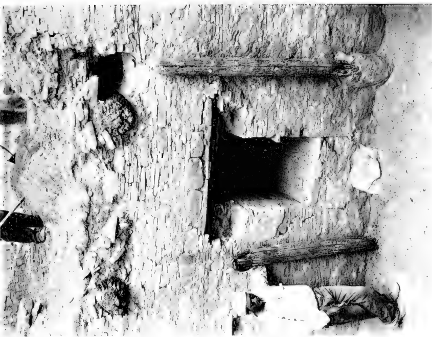
B. Partially blocked east door in Room 43A with slab step and, at either side, props for ceiling beams.
