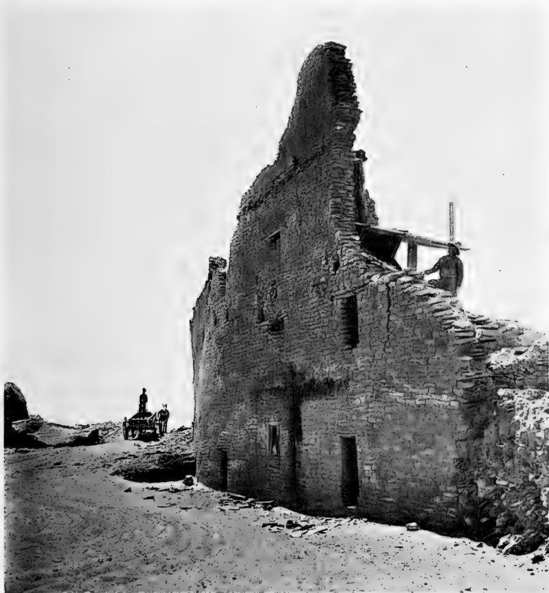
FIG. 71.—Extensive repairs have been made to strengthen the shattered walls of prehistoric Pueblo Bonito and preserve its masonry for future generations. Four stories are evident in this particular view. (Photograph by Neil M. Judd. Courtesy of the National Geographic Society.)
