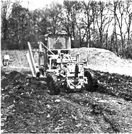
Fig. 2. Raw sludge is mixed with wood chips in the ratio of three parts wood chips to one part sludge.
