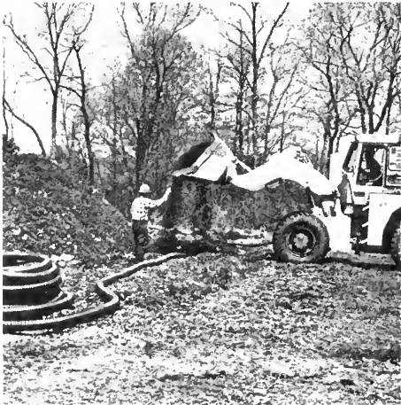
Fig. 4. Four inch perforated pipe is placed on the bed and covered with four inches of wood chips.
