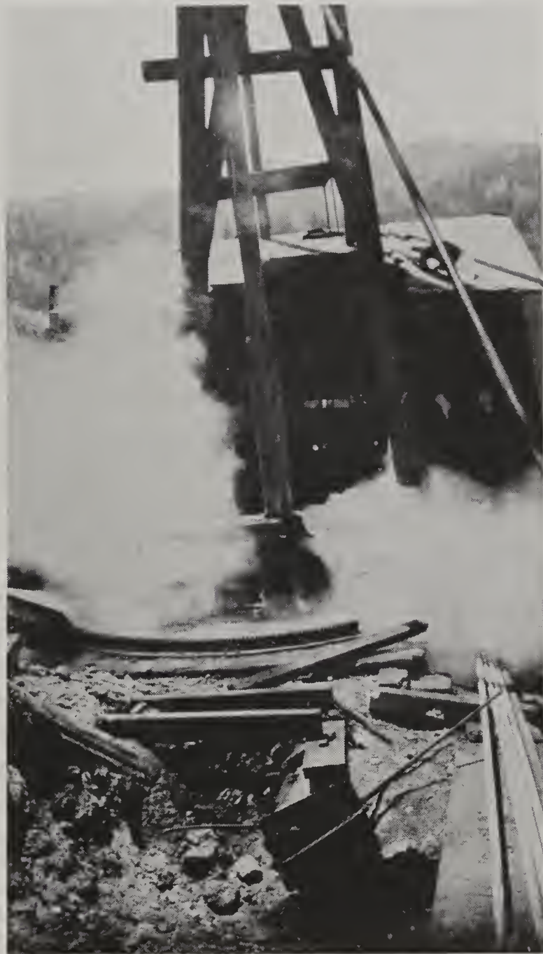
FIG. 20—A plank across mouth of casing, weighted with drill rod weighing about a ton, fails to “hold down” steam, 1922.
