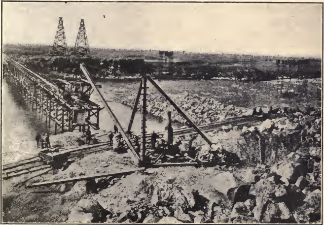
FIG. 38.—Showing derrick handling skips, and cableways in action; also showing double trestle from which earth was dumped in the back-filling, Minidoka project, Idaho (U. S. Reclamation Service).
