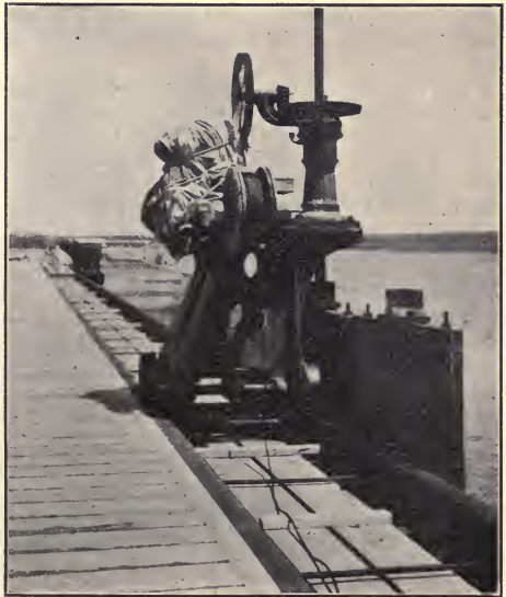
FIG. 30.—Milner Dam, showing lifting apparatus operated by electric motor.
