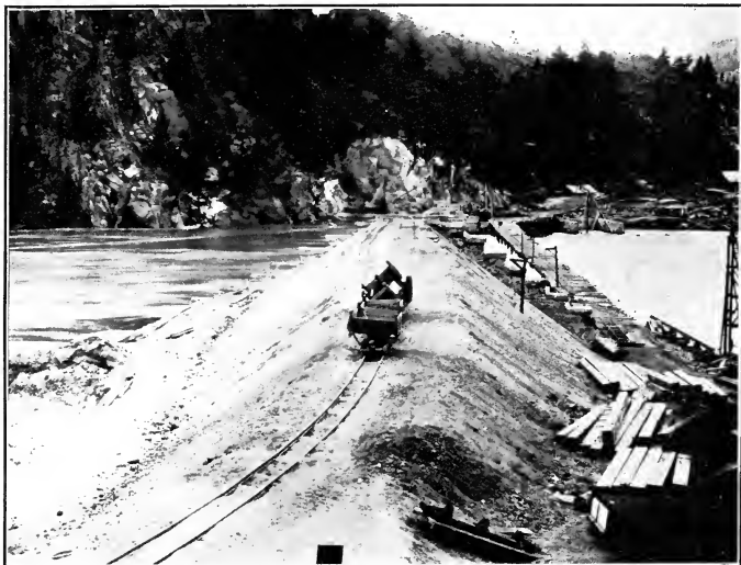
FIG. 1.—METHOD OF CONSTRUCTING EARTH FILL AT END OF CRIB DAM, CANYON FERRY DAM, MONT.
