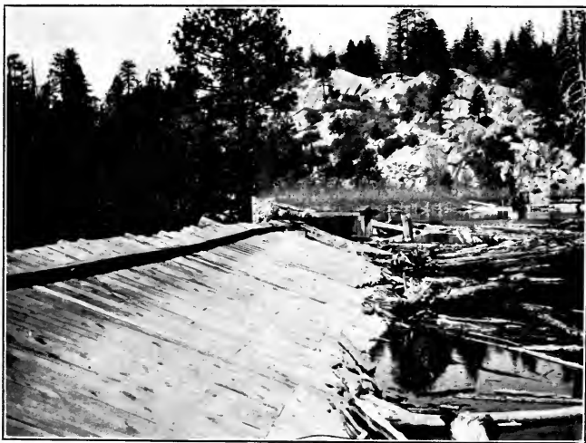
FIG. 2.—PLANKING ON UPSTREAM FACE OF MIDDLE DAM, SOUTH FORK STANISLAUS RIVER, CAL.
