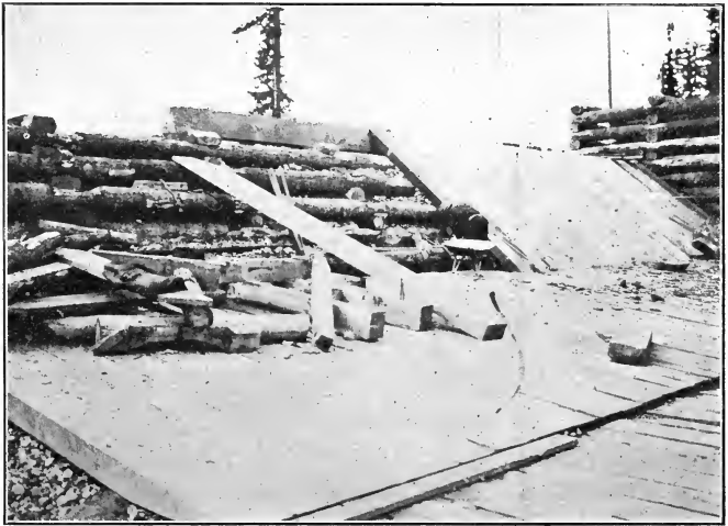
FIG. 12.—Lake Keechelus Dam, apron and spillway under construction, crest log in place and apron completed on east end.
