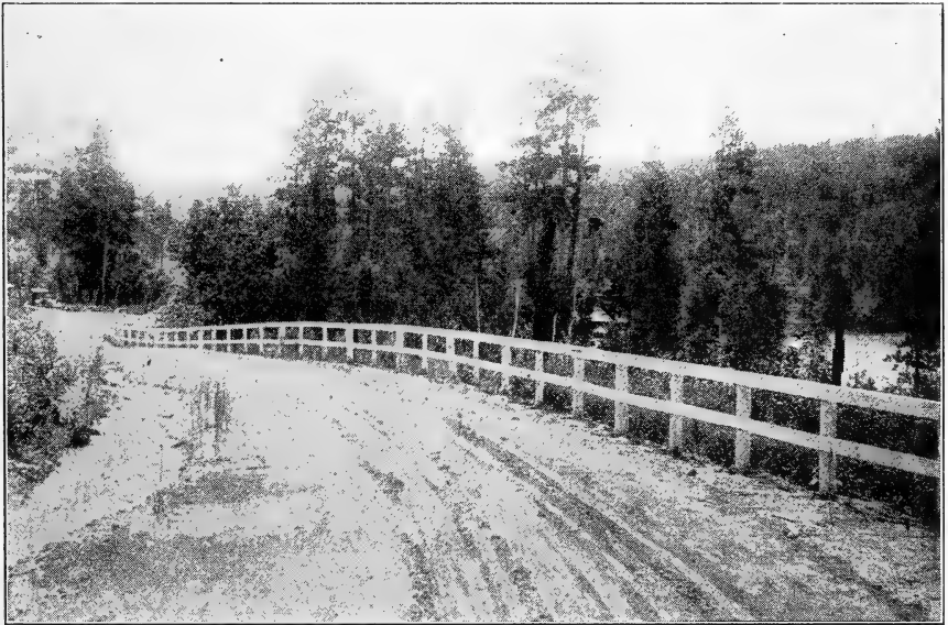
FIG. 89. As It Is. Auto Road in Itasca State Park.
