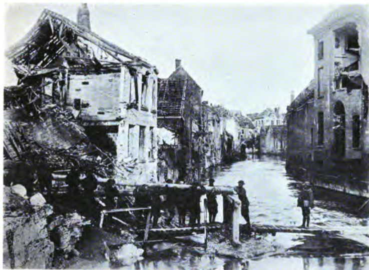
Placing abutment for bridge over canal in town of Audenarde. City was badly damaged by shell fire.
