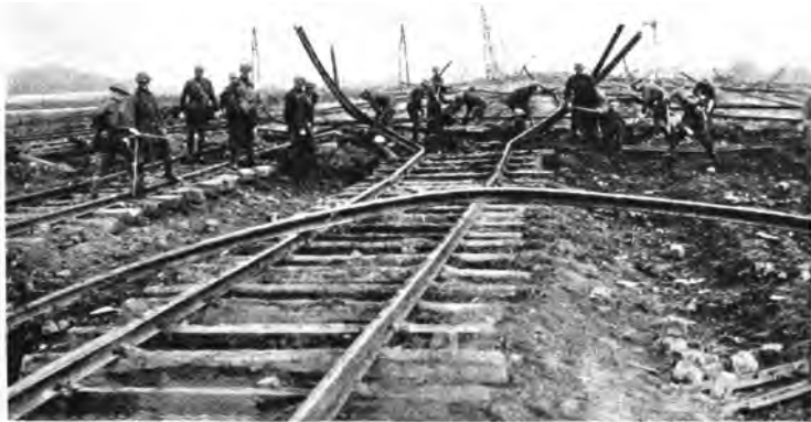
View of destroyed railroad tracks at Waereghem, Belgium. These tracks were destroyed by mines before the Germans retreated from the city. Men working in picture are from Company A, 316th Engineers.
