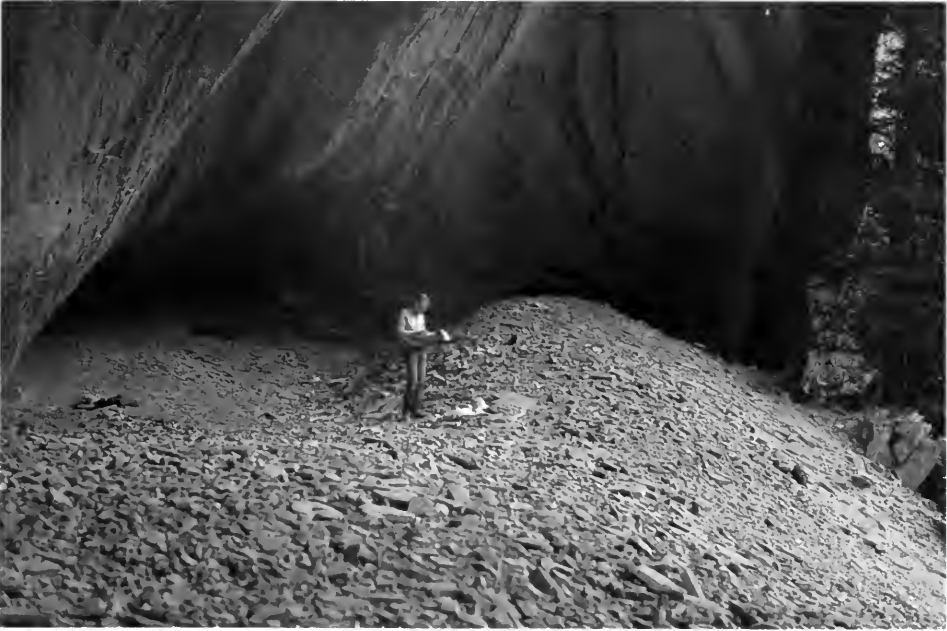
Figure 5-13. Cave with an unstable roof.
