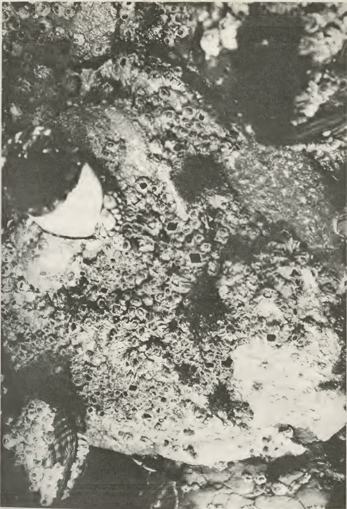
Figure 13B. Dense growth of Balanus glandula and Chthamalus spp. on the concrete surface, January 1972, one year after the oil spill. Plastic pipe is at the upper left side.
