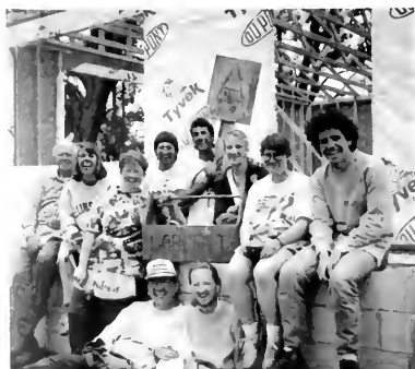
Over the '91 spring break, students in the Habitat for Humanity project and faculty advisor Jerrell Habegger helped build a house for the financially underprivileged in St. John's Island, SC.
