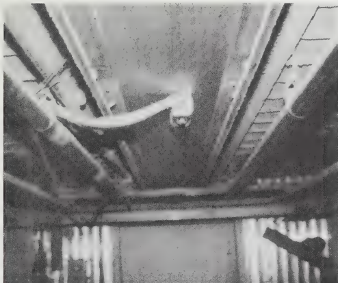
Figure 27 - Black iron pipe radiator
