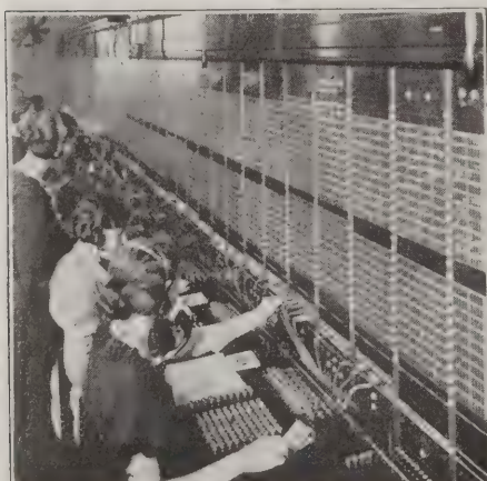
Central Machine Switching Cutover—Semi-Mechanical "A" Switchboard.
