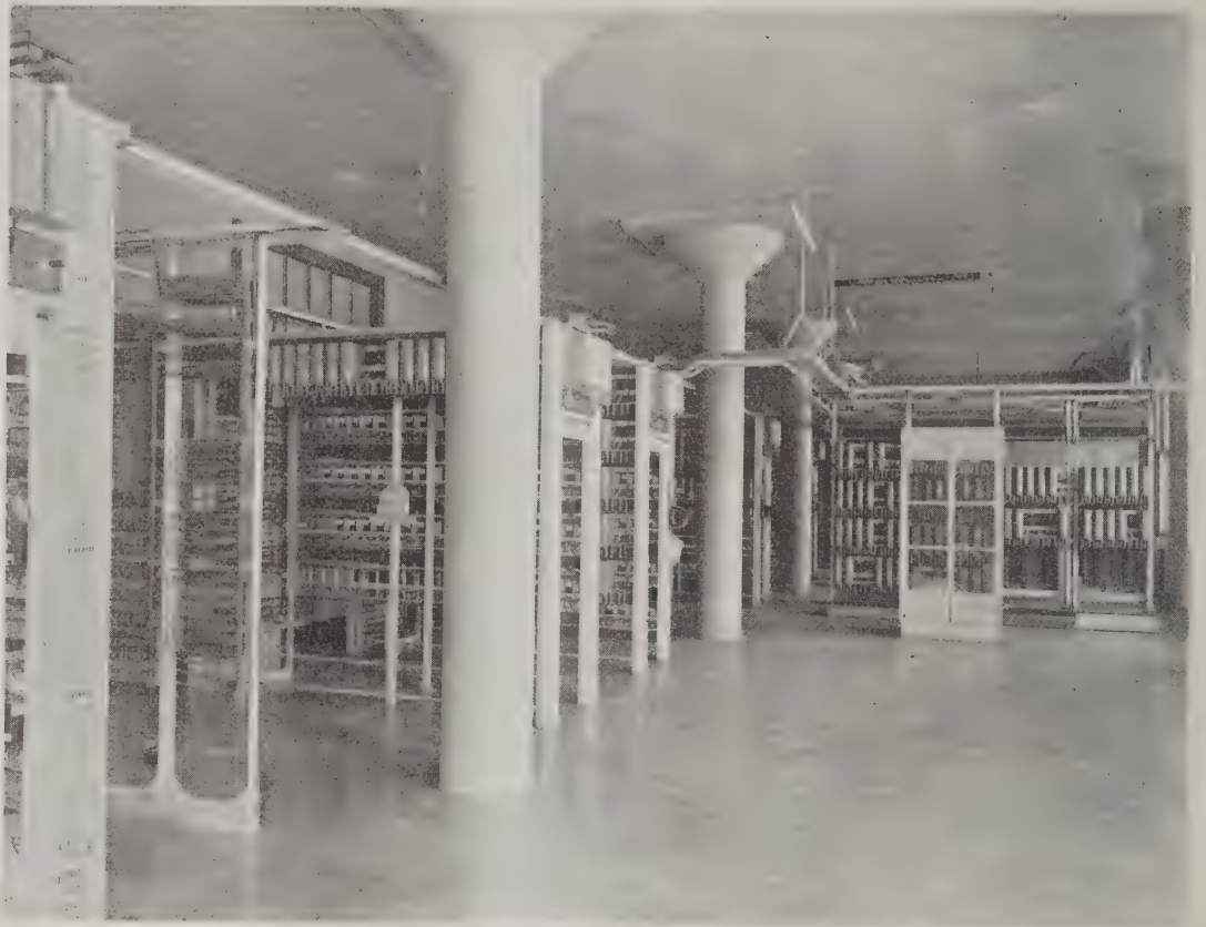
The Marion County Telephone Company, operating exchanges at Marion, Waldo, Green Camp, and Morrall, Ohio, believes in modern equipment. Not a single manual telephone is connected to any of their exchanges, all of which are of the Strouger Automatic type. Above is shown the Marion switchroom.
