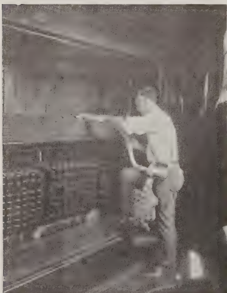
Cleaning the Multiple Cable in the Rear of the Switchboard With the New Vacuum Cleaner.
