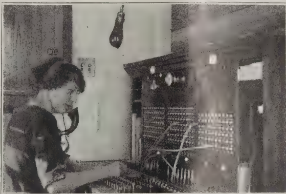
Newly Installed Switchboard in New Exchange Building of Northeastern Telephone Co., Walthill, Nebr.
