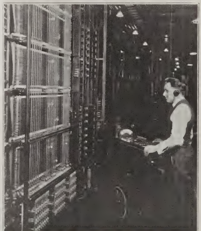
Final Frame, Showing "Tea Wagon" Test Set in the New CENTRAL Office in Chicago.
