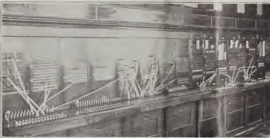
View of the New Marysville Switchboard Just Preparatory to the Cut-Over.
