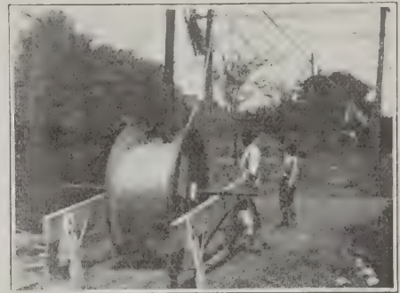
Simple and Inexpensive Cable Reel Mounting.
