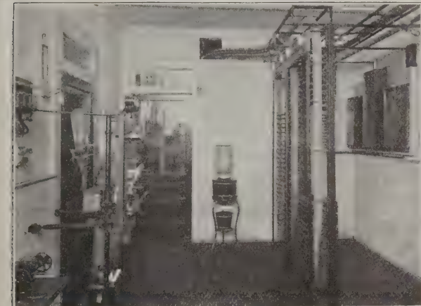
Left: Neatly Arranged Terminal Room.
