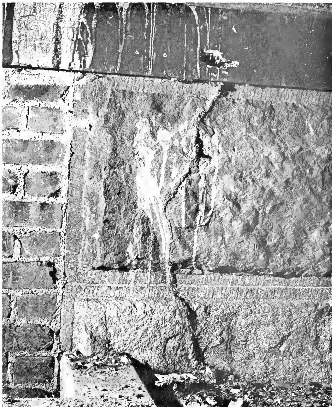
Figure 2. Termites constructed this shelter tube from wood to the ground in a partly excavated area, formerly an exterior wall.
