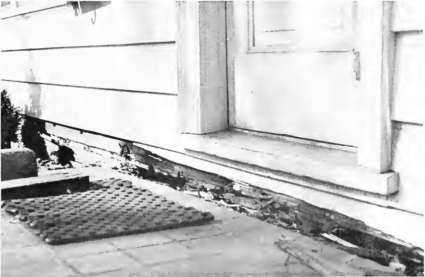
Figure 3. Direct contact between the sill and the earth fill under masonry porches or steps is an invitation to termite infestation. Part of the masonry floor has been removed to make repairs.
