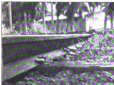
FIG. 2.—BETWEEN THE SPIKE SHOWN NEAR THE CENTER OF THE ILLUSTRATION AND THE RAIL FLANGE A HEAVY INCRUSTATION HAS FORMED
