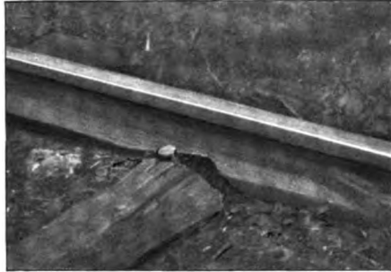
FIG. 5.—IN THIS CASE THE RAIL FLANGE WAS EATEN ENTIRELY THROUGH. THE SPIKE SHOWN IS A NEW ONE, PLACED FURTHER ALONG ON THE EDGE OF THE TIE
