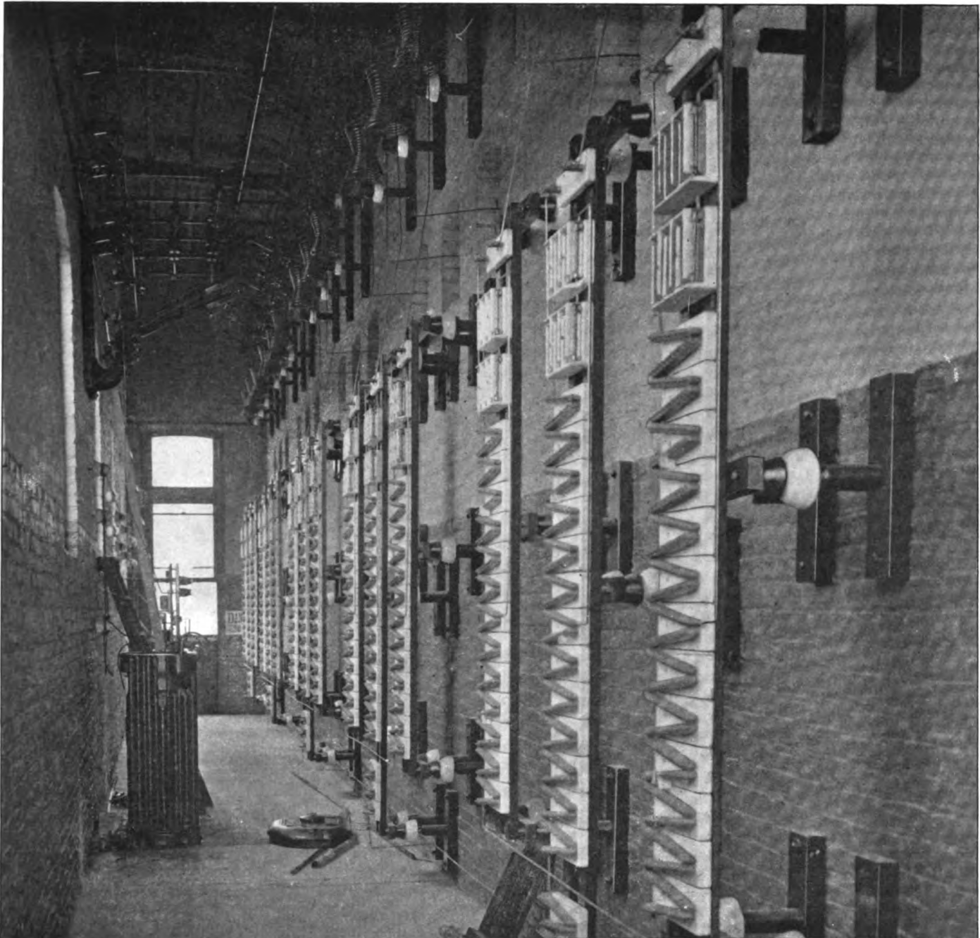
FIG. 11.—THE LIGHTNING ARRESTER ROOM IN THE SUB-STATION AT NEWFIELD, SHOWING ALSO THE DISCONNECTING SWITCHES
