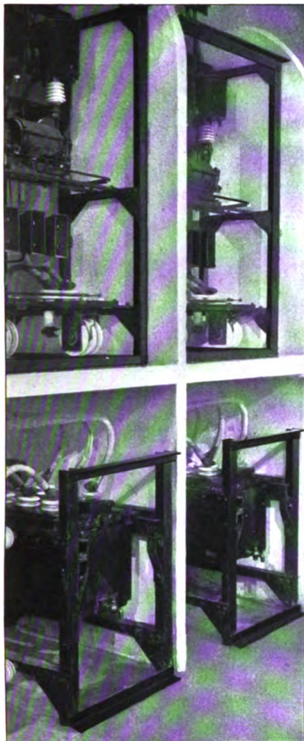
FIG. 7.—OIL SWITCHES AND TRANSFORMERS FOR SUPPLYING CURRENT TO SWITCHBOARD INSTRUMENTS IN THE PLANT AT MONTEREALE
