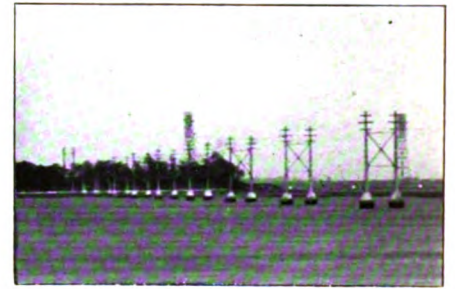
FIG. 12.—PART OF THE TRANSMISSION LINE FROM MONTEREALE TO VENICE. FOUR THREE-PHASE CIRCUITS ARE MOUNTED ON DOUBLE POLES
