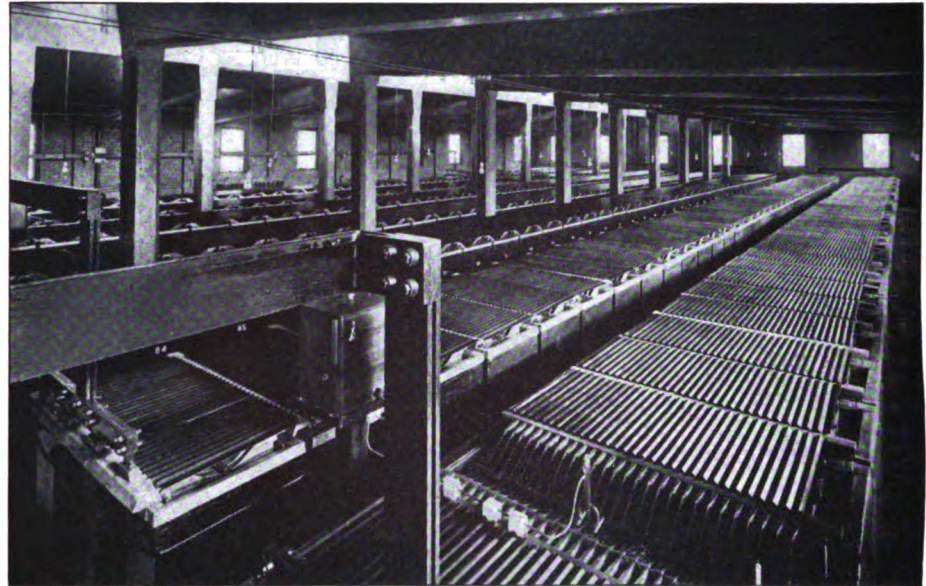
FIG. 11.—IN THE SUB-STATION AT HAMMEL, 300 CELLS OF 3200 AMPERE-HOURS CAPACITY ARE INSTALLED WITH TWO 162-KW. BOOSTERS TO TAKE CARE OF THE LOAD FLUCTUATIONS ON THE ROCKAWAY BEACH LINE
