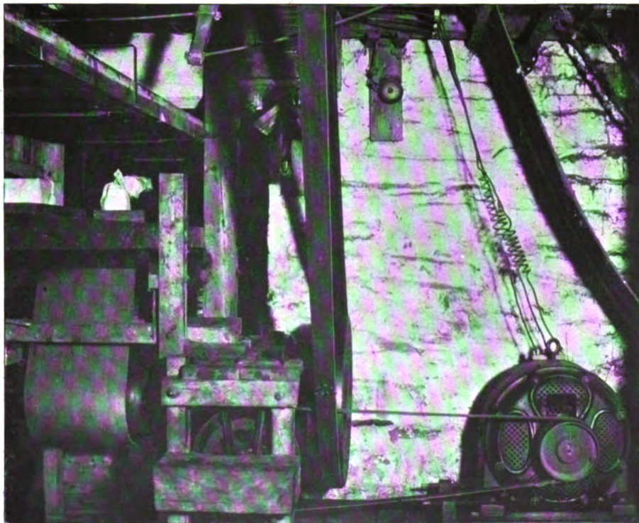
A MOTOR DRIVING A PARCELS CONVEYOR, WHICH TAKES PARCELS FROM SALESROOMS TO ASSORTING SECTION PRIOR TO SHIPMENT. THIS MOTOR ALSO DRIVES A BARREL HOIST
