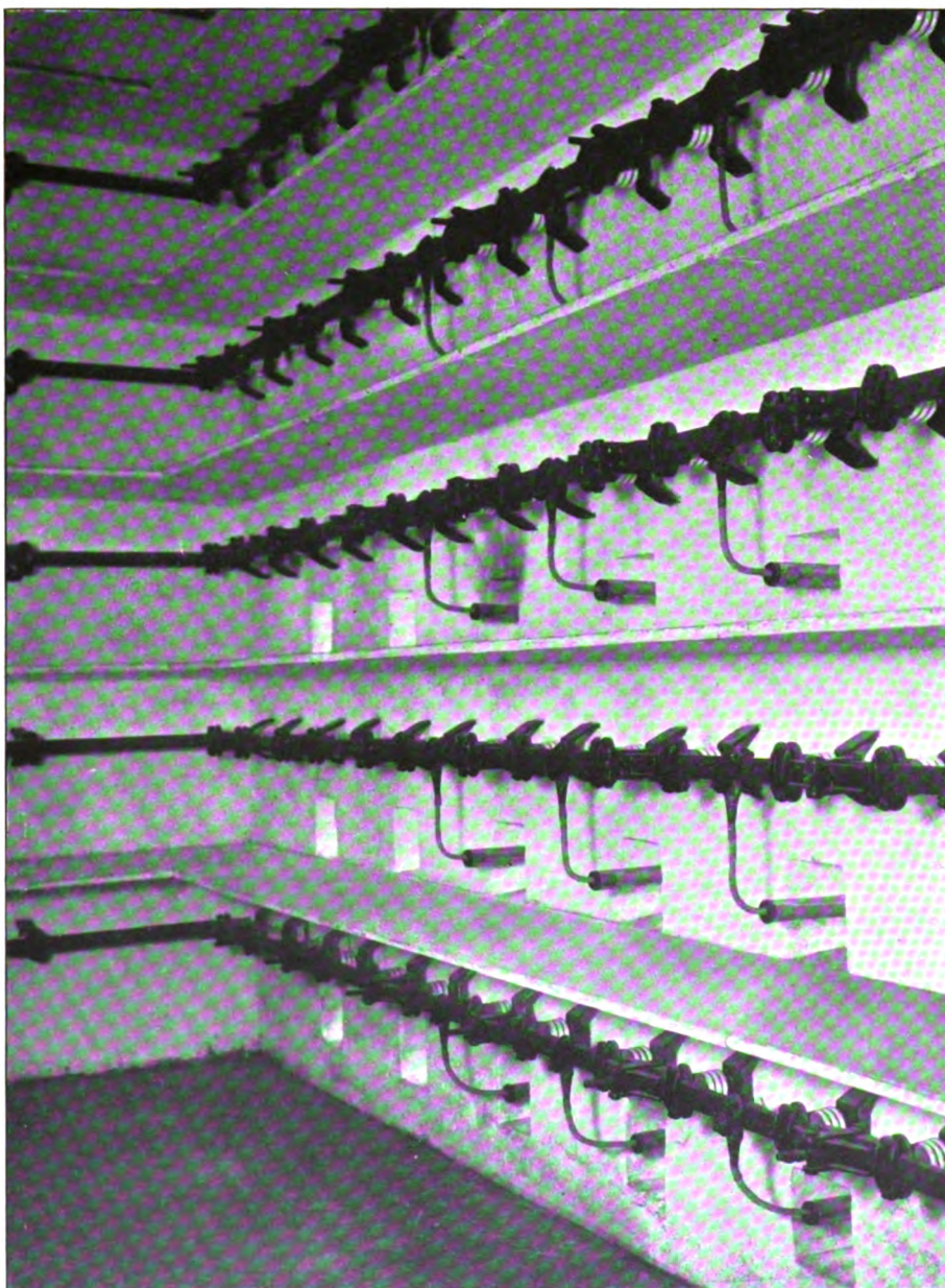
FIG. 5.—BUS-BARS IN THE VENICE SUB-STATION, WHICH RECEIVES CURRENT FROM THE POWER PLANT AT MONTEREALE
