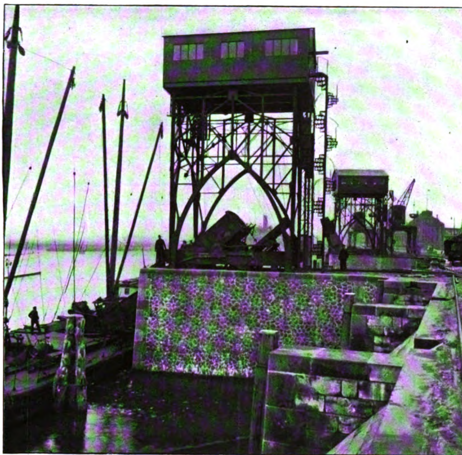
FIG. 2.—FOR LOW-WATER LEVELS, THE TIP IS OPERATED AUTOMATICALLY BY THE WEIGHT OF THE LOADED CAR
