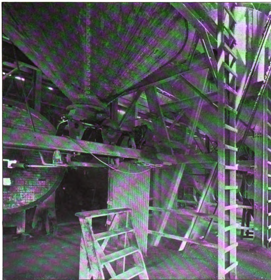
A COAL FEEDER OPERATED BY AN INDUCTION MOTOR
