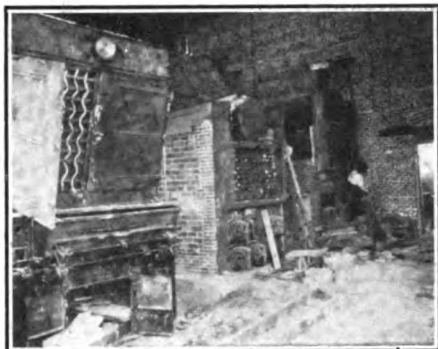
FIG. 2.—INTERIOR OF THE BOILER HOUSE.
