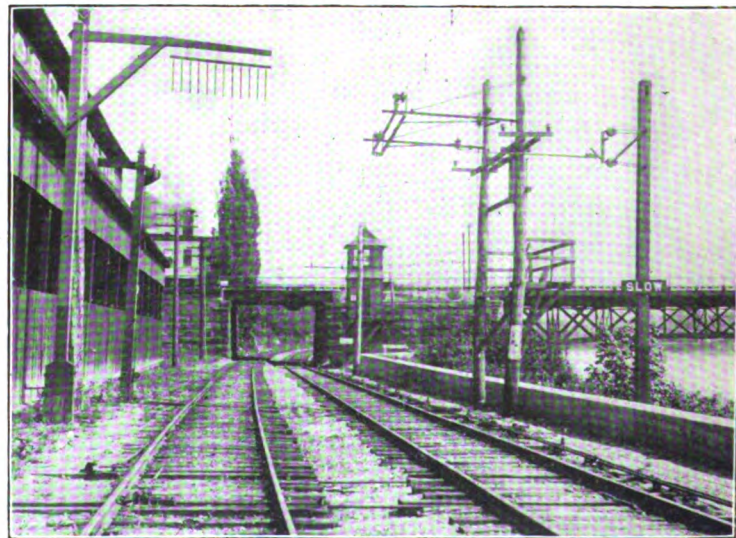
OVERHEAD CONSTRUCTION AT CLARISSA STREET BRIDGE, ROCHESTER—SHOWING TROLLEY SECTION INSULATOR AND BRIDGE WIRING.
