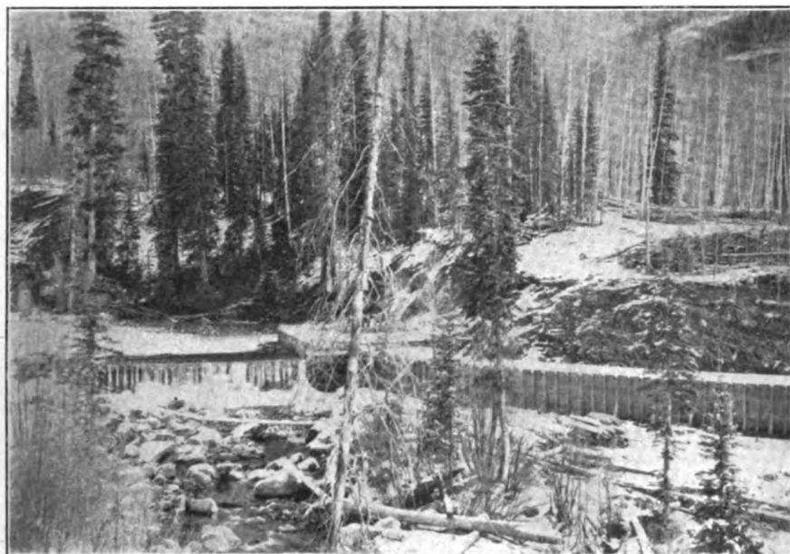
FIG. 1.—THE DIVERTING DAM AND HEADGATE AT CASCADE CREEK, A TRIBUTARY OF THE ANIMAS RIVER IN COLORADO. THE PRESENT 6000-H. P. DEVELOPMENT OF THE ANIMAS POWER & WATER COMPANY UTILIZES ONLY THE WATERS OF THIS CREEK
