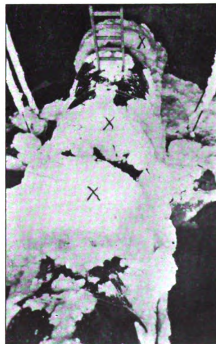
FIG. 6.—FRAZIL AND ANCHOR ICE FORMATION ON A TURBINE PENSTOCK. NOTE THE FORMATION, ABOUT 14 INCHES DEEP, OVER THE WHEEL ENTRANCES, MARKED WITH A CROSS, AND ALSO THE FRAZIL CLINGING TO THE RODS
