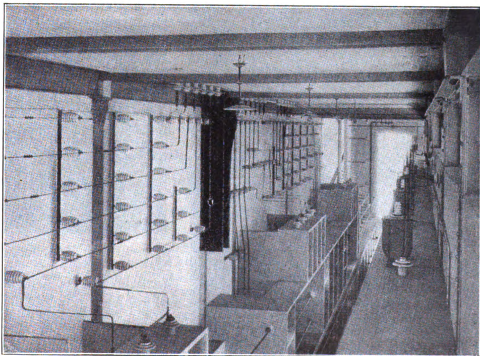
Fig 11—27,000-VOLT BUS BARS.
