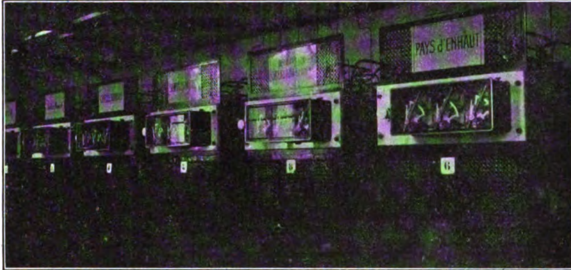
Fig. 9.—EUROPEAN (ALIOTH) CABINET, HAND OPERATION, MONTBOVEN STATION
