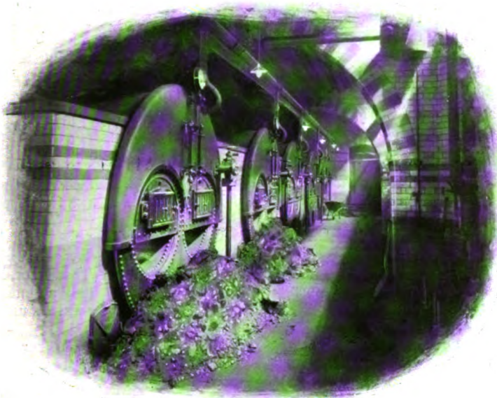
THE BOILERS AT THE PRUDENTIAL COMPANY'S OFFICES.
