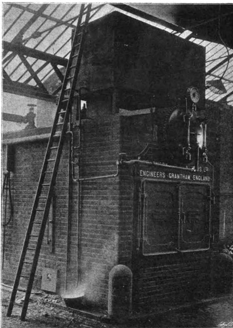
THE ST. PANCRAS BOILER.
