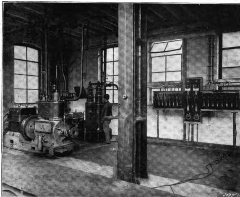
GENERATING PLANT FOR SHOP DRIVING.
