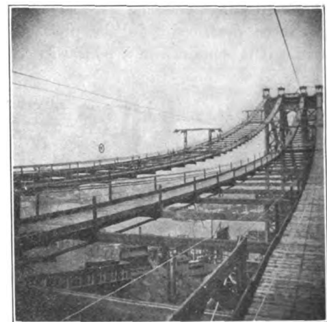
CABLE-HAULING ON THE NEW MANHATTAN BRIDGE. A VIEW FROM THE TOP OF THE ANCHORAGE.
