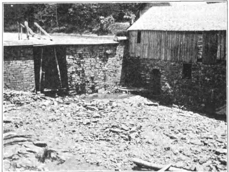
A VIEW TAKEN BELOW THE DAM, SHOWING A PART OF THE POWERHOUSE ON THE RIGHT.
