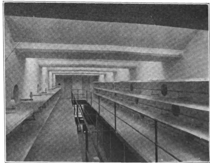
FIG. 21.—BUS-BAR ARRANGEMENT AT LOMAZZO.
