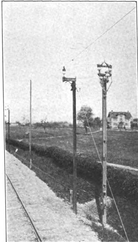
HORN SECTION-SWITCH AND DEAD-END OF ONE TROLLEY SECTION — SEEBACH-WETTINGEN SINGLE-PHASE RAILWAY.
