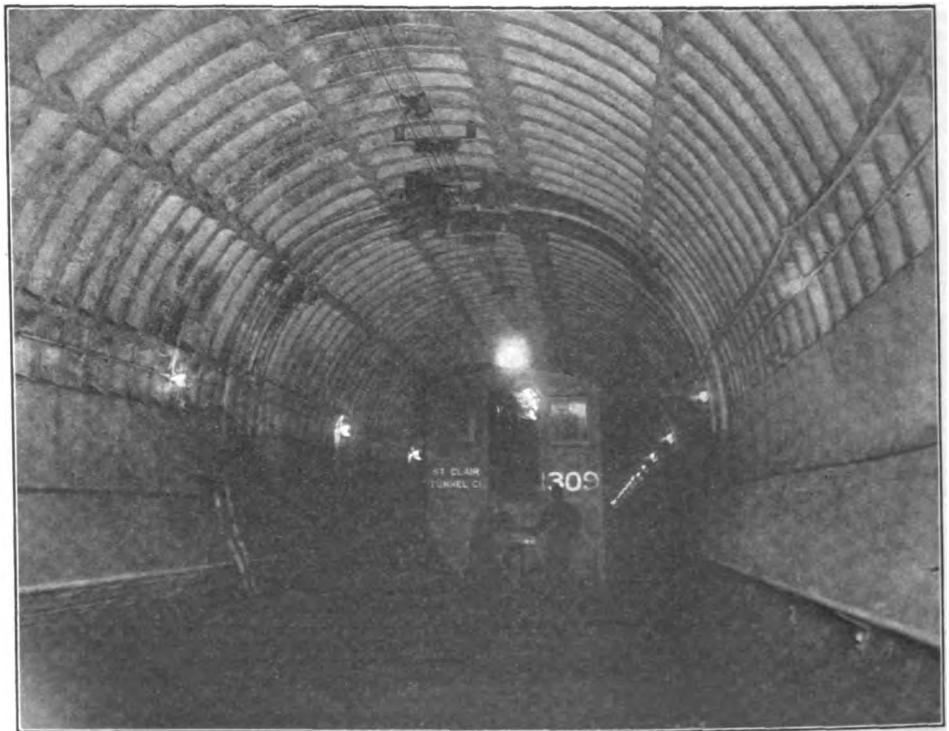
ELECTRIC LOCOMOTIVE IN THE ST. CLAIR TUNNEL, SHOWING THE INTERSECTION OF THE VERTICAL SHAFT THROUGH WHICH ARE BROUGHT THE FEEDERS FROM THE POWER HOUSE.
