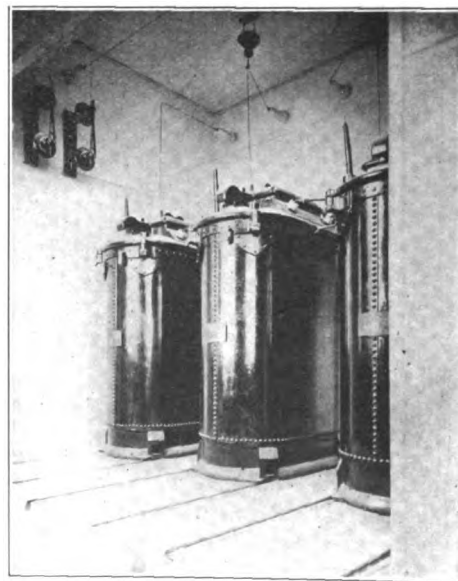
A BANK OF THREE HIGH-TENSION TRANSFORMERS OF BRILLANNE HYDROELECTRIC PLANT.
