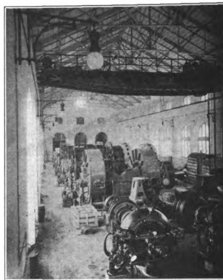
INTERIOR VIEW OF BRILLANNE HYDROELECTRIC PLANT.
