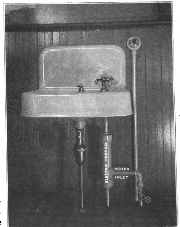
FIG. 2.—GRINNELL INSTANTANEOUS WATER HEATER IN WATER INLET TO WASH BASIN.
