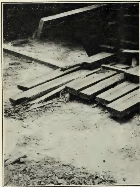
FIG. 35.—Projecting ends of lumber which have decayed by coming in contact with the ground.
