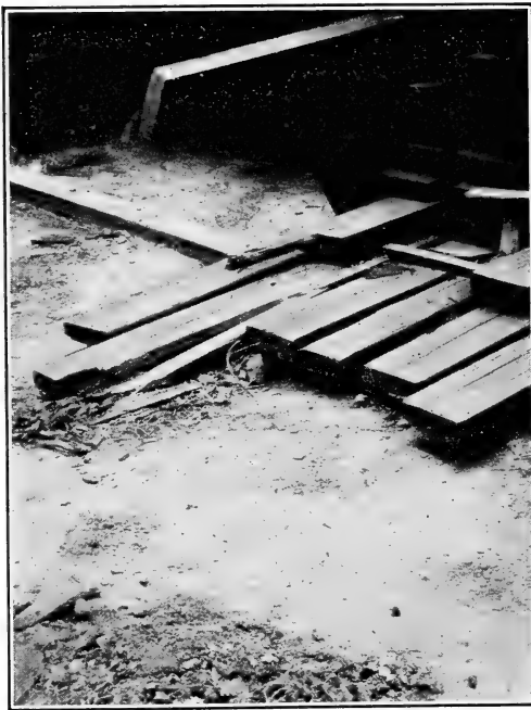
FIG. 35.—Projecting ends of lumber which have decayed by coming in contact with the ground.
