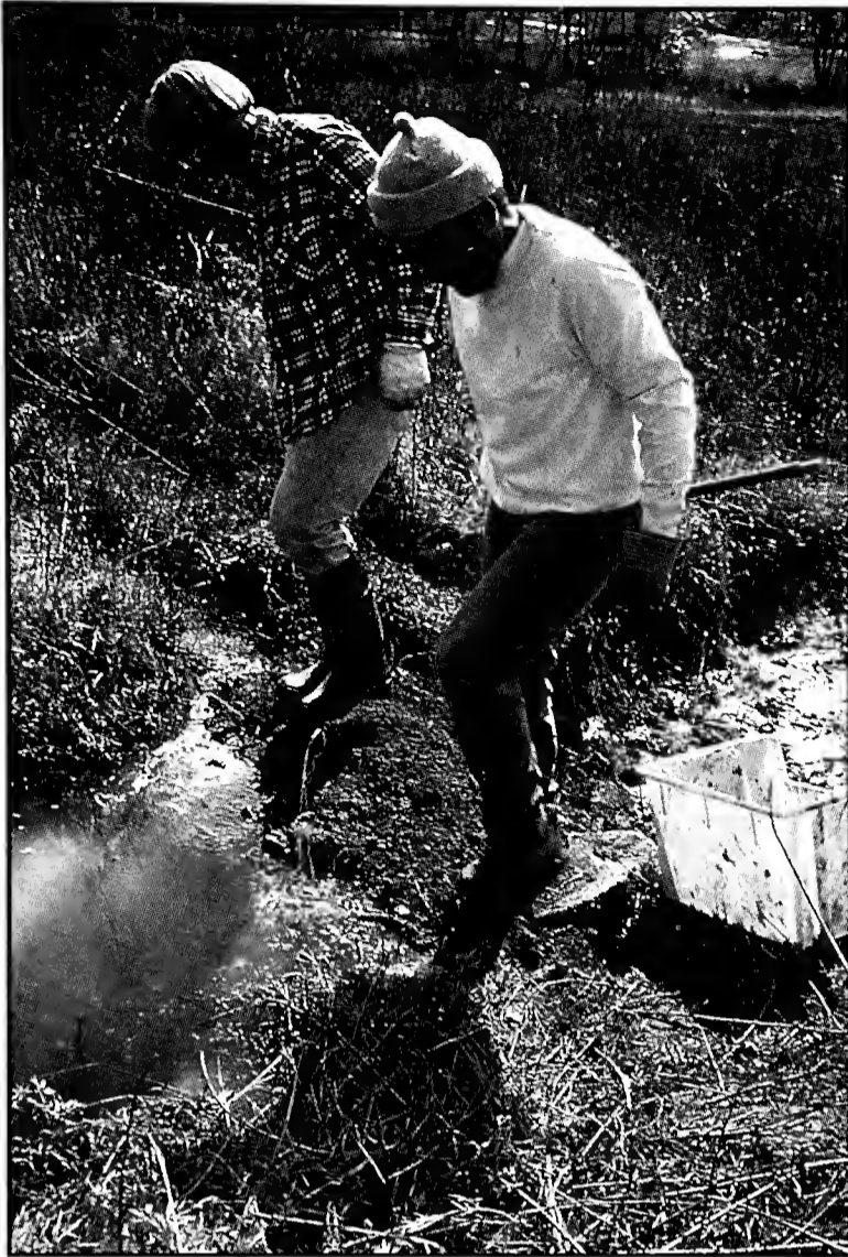
Ron Determann and Malcom Hodges restore hydrology to a bog by filling a ditch.
