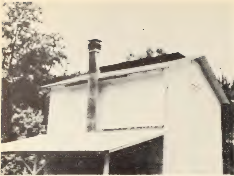
Figure 21.--Many of the modern type flue-cured curing barns are heated by oil or gas.
