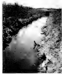
Ditch made with dynamite. The ditch is being used for the power plant.
