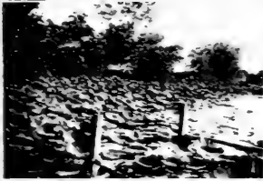
Debris piled up after clearing of brush and trees from the site of the new dam. The debris is being used for fuel in the power plant.
