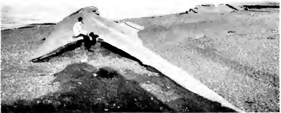
Concrete sea wall broken by tide of Dec. 31st, 1921
