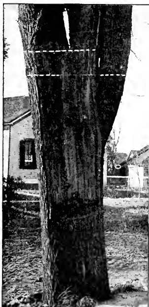
Photo 39 A Bolt is Needed.
