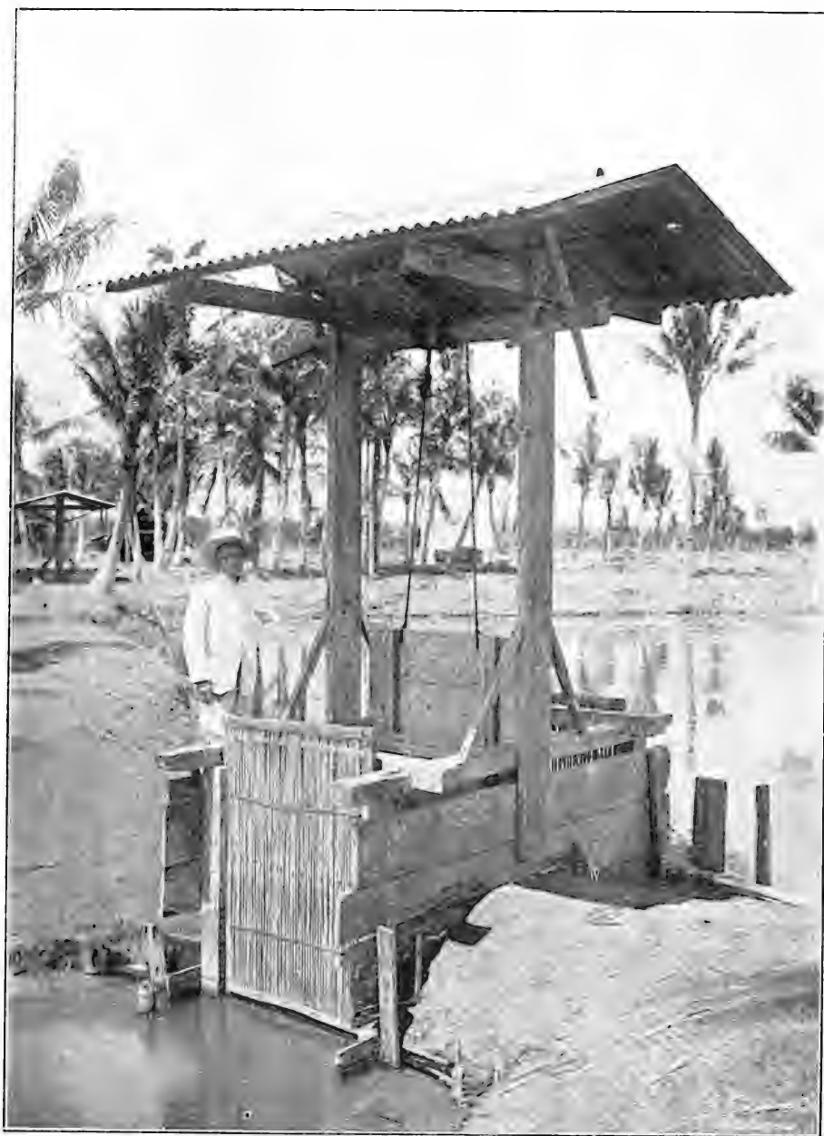
Photo no. 1. (Taken in 1915). Little sluice gate connecting two Batavia sea-fish-ponds, Pondsysteem of Ang Sun Hian, Groningsche weg near Kampong Fiuit (cf. Map I).
