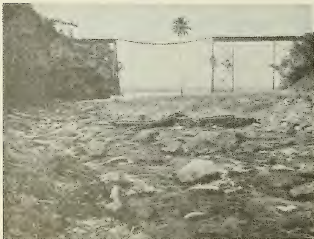
Figure 64. Tsunami damage to railroad trestle on Kolekole Stream, Island of Hawaii (from Shepard, MacDonald, and Cox, 1950).
