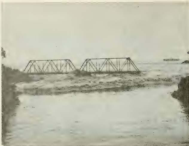
Figure 63. Tsunami damage to railroad bridge on Wailuku River, Hilo, Hawaii (photo by Shigeru Ushijima; from Shepard, MacDonald, and Cox, 1950).
