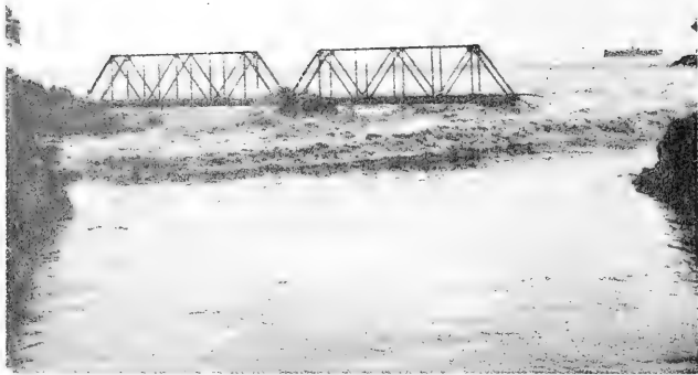
Figure 63. Tsunami damage to railroad bridge on Wailuku River, Hilo, Hawaii (photo by Shigeru Ushijima; from Shepard, MacDonald, and Cox, 1950).
