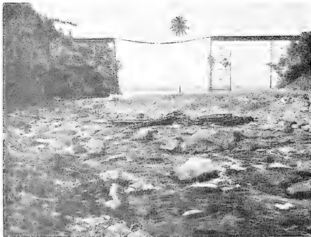
Figure 64. Tsunami damage to railroad trestle on Kolekole Stream, Island of Hawaii (from Shepard, MacDonald, and Cox, 1950).
