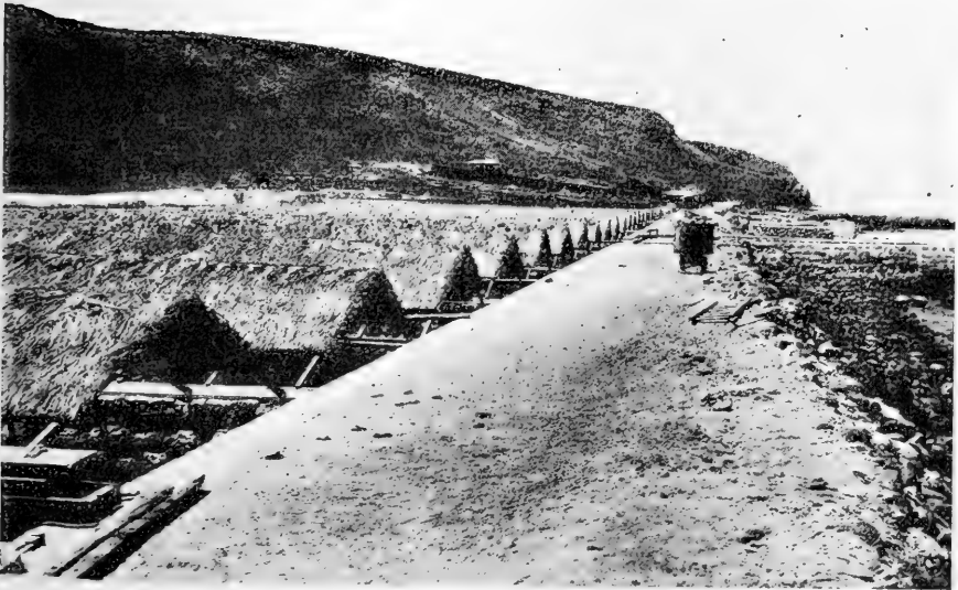
Fig. 28. Thatched roofs over the cross-sections of the canal; the open Bay on the right.
