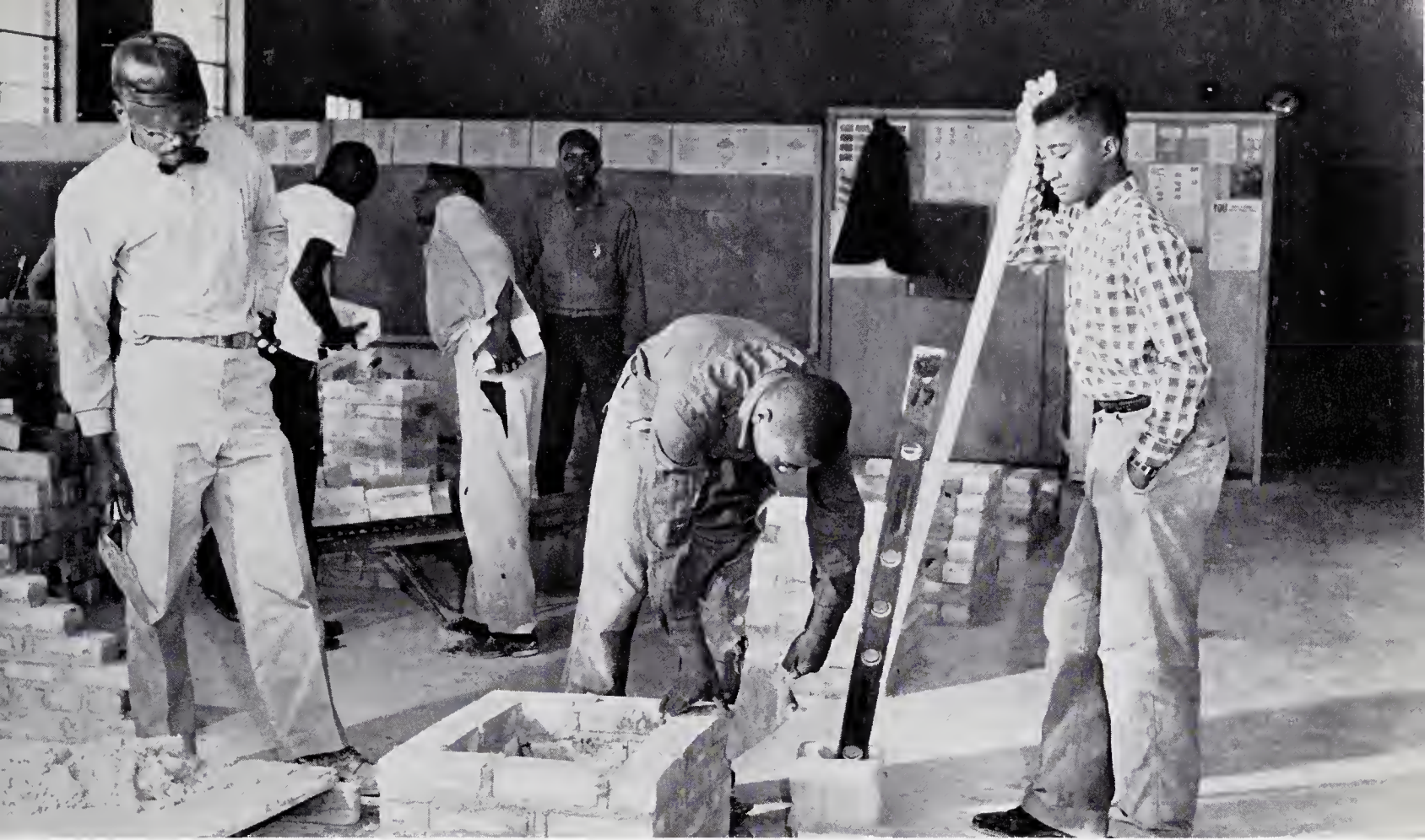
Mr. Wade, (trowel in hand) sees to it that bricks are carefully placed
