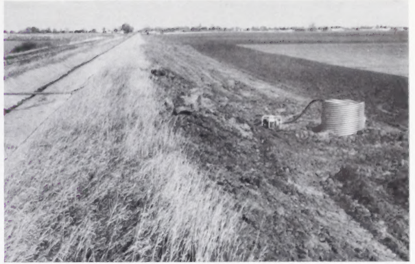
Portable pump at manhole (picture taken before submersible pump was installed).
