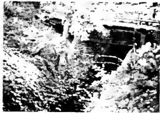
Glen Echo Creek, Oakland, California. A dry rock wall was hand built by the Richmond Boulevard Association in Oakland.
