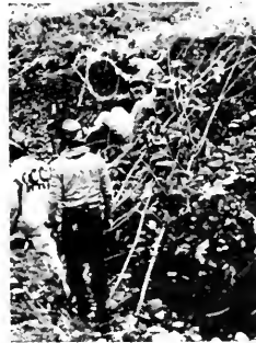
Lindo Channel, Chico, California. Members of the California Conservation Corps are securing dead vegetation "deflectors" to divert flows away from an eroding bank.
