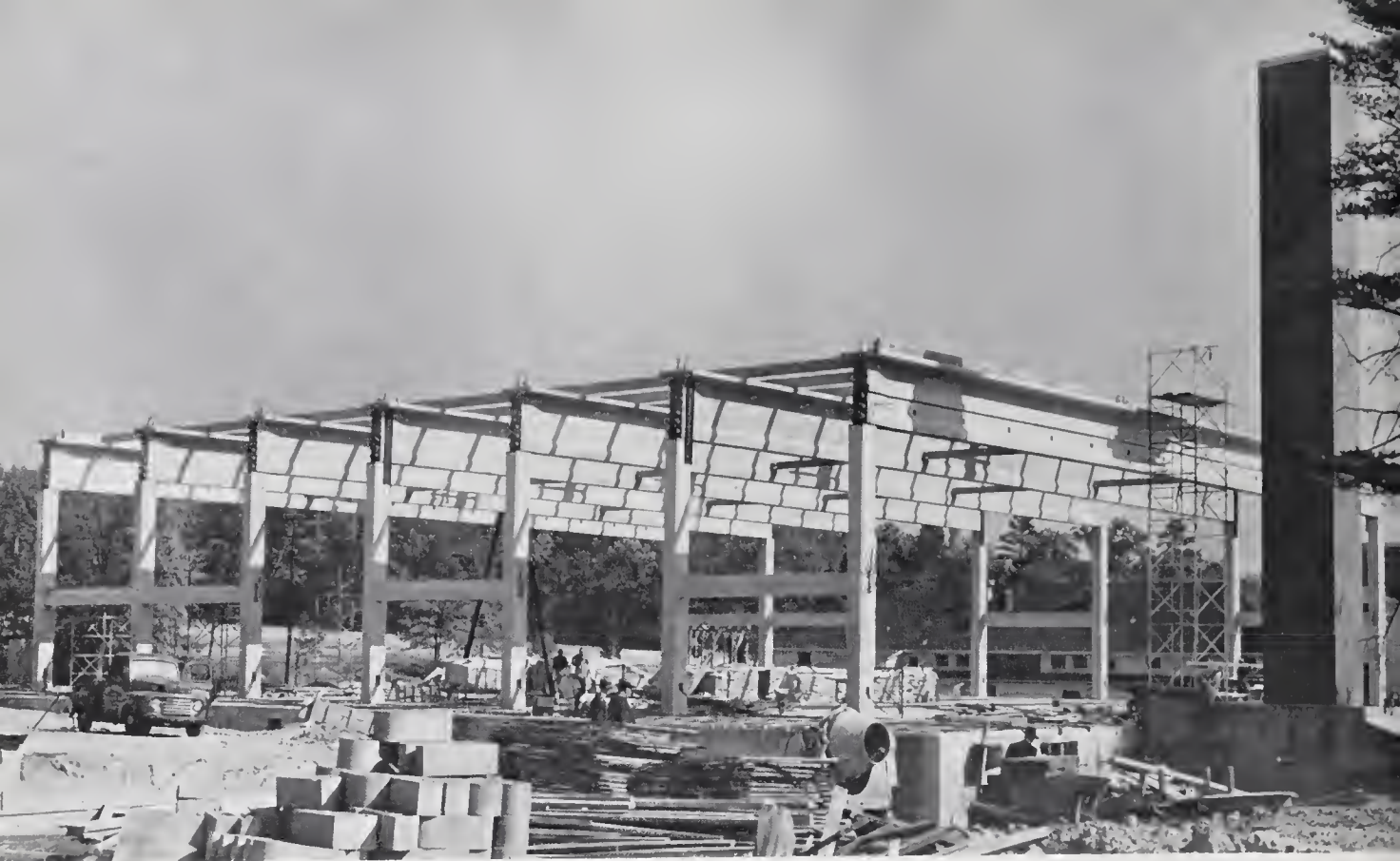
All is quiet in this picture of these 125-foot pre-stressed concrete beams of the new gym. But as this longest span of this type yet used in the United States went up into place last October, hordes of spectators surrounded the scene of activity.
