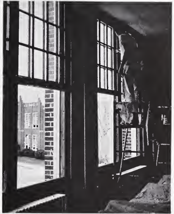
NEW COAT of paint for GHS means brighter rooms for students, a year's work for painters.
