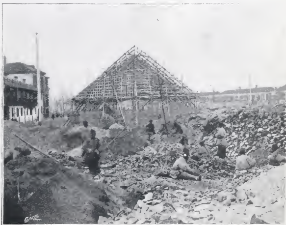
CHINESE BUILDING OPERATIONS.—"THE SHAPE OF THE STRUCTURE IS FASHIONED OUT OF LONG BAMBOO RODS." [Photo.
