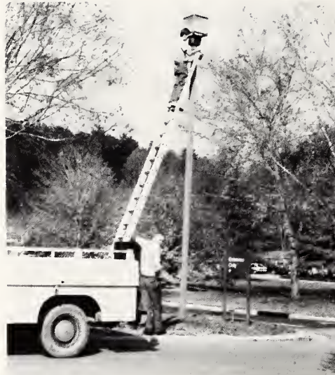
Maintenance work never ends. Here, Mr. Eugene Souther supervises as Mike Severt checks a campus street light.
